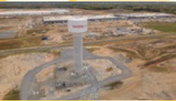
Toyota Battery Manufacturing, North Carolina社(米国)
