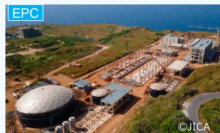
EPC Senegal – Desalination plant
