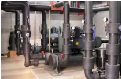
Geothermal heat pump at Tianjin Fengtian Steel Process Co., Ltd. (China)
