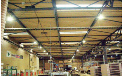
LED lighting at Toyotsu-new Pack
