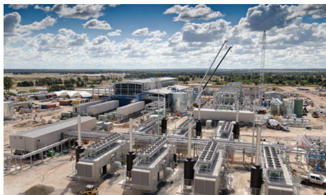
Construction of a water processing plant to minimize environmental impact (Photo shows plants under construction in neighboring mining sector)
