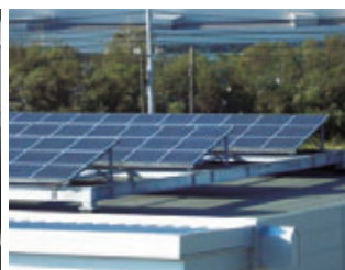
Solar power generation (Hokkaido Branch)
