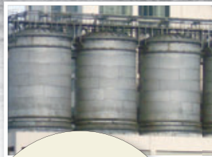
PET polymer facility
