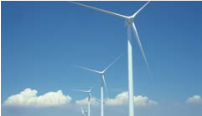
Wind power generation
