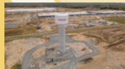
Toyota Battery Manufacturing, North Carolina (U.S.)
