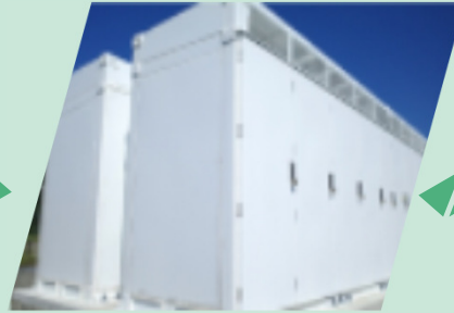
AI-based grid storage battery control system (ReERa)
