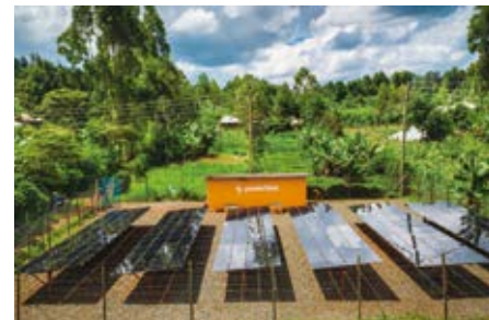
A mini-grid installed in a non-electrified region of Kenya
