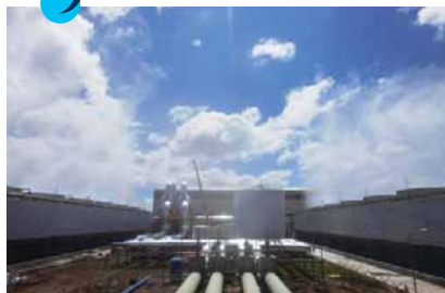
Kenya's largest geothermal power project
